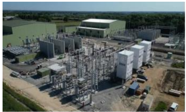
Converter Station, Dogger Bank
